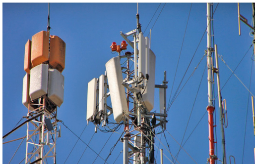
Figure 3. Base transceiver station (BTS)
